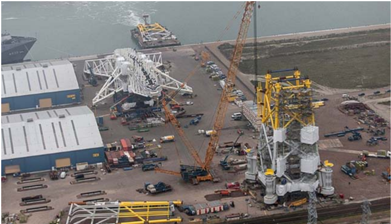
Seen in the Scaldiahaven Vlissingen several construction activities Photo: Hans van der Linden www.aerolin.nl @AerolinPhotoBV ©
