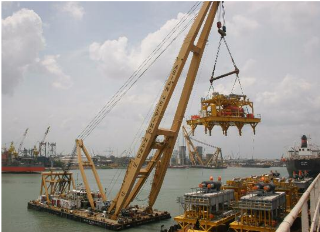
Above seen the sheerlegs ASIAN HELPING HAND III installing a compressor onboard the Lewek FPSO 1 in Singapore
