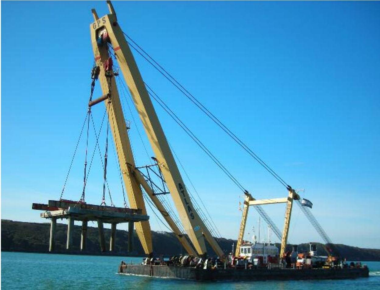
The sheerlegs GPS Atlas seen working at Milford Haven South Hook Project.
