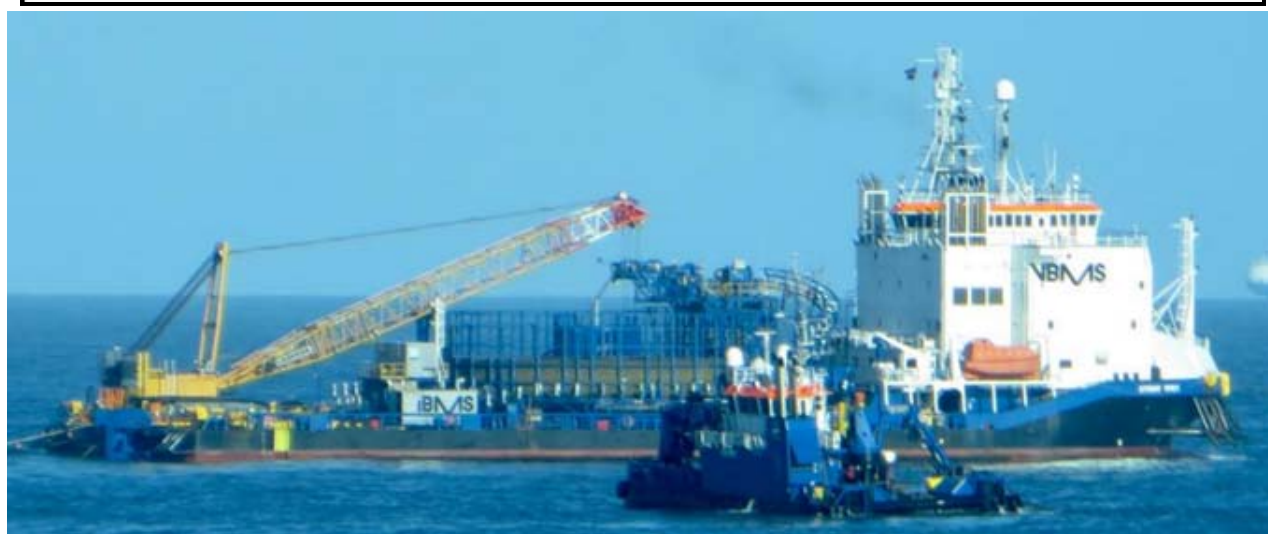
STEMAT SPIRIT and ANNA B. laying cables at the Dudgeon Offshore Wind Farm, UK Northsea.
