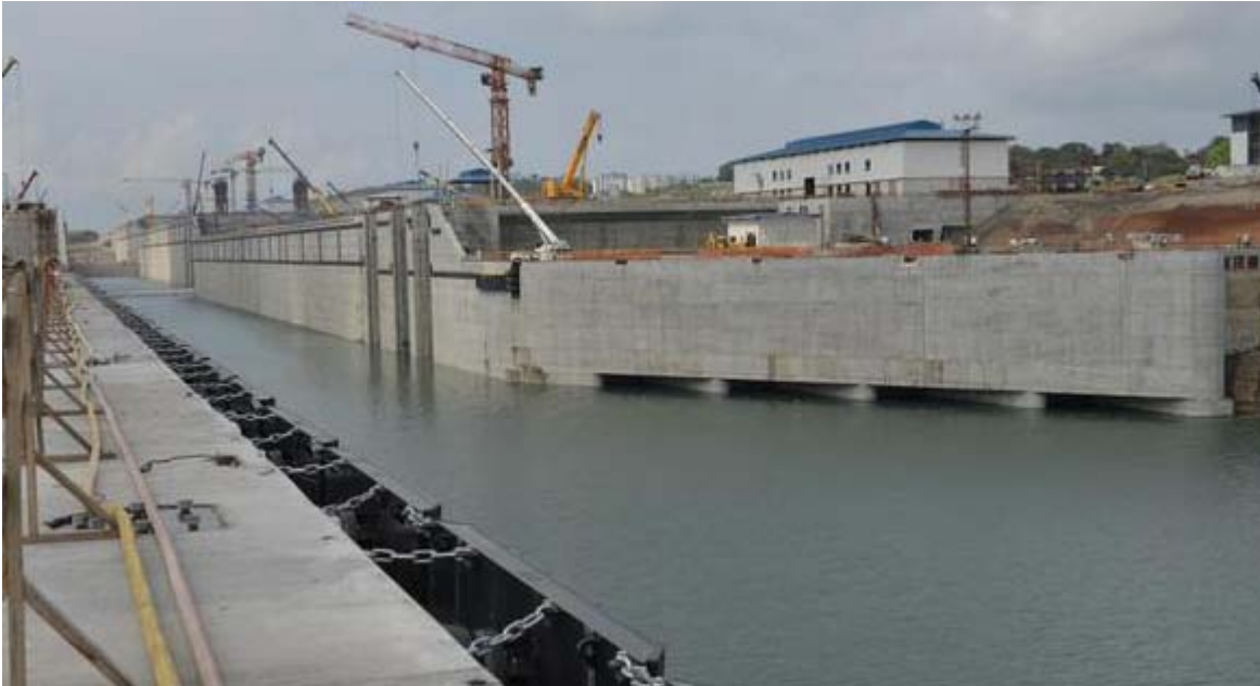
Ongoing filling of the lower chamber of the new Atlantic locks at the Panama Canal Expansion . Photo : Panama Canal
