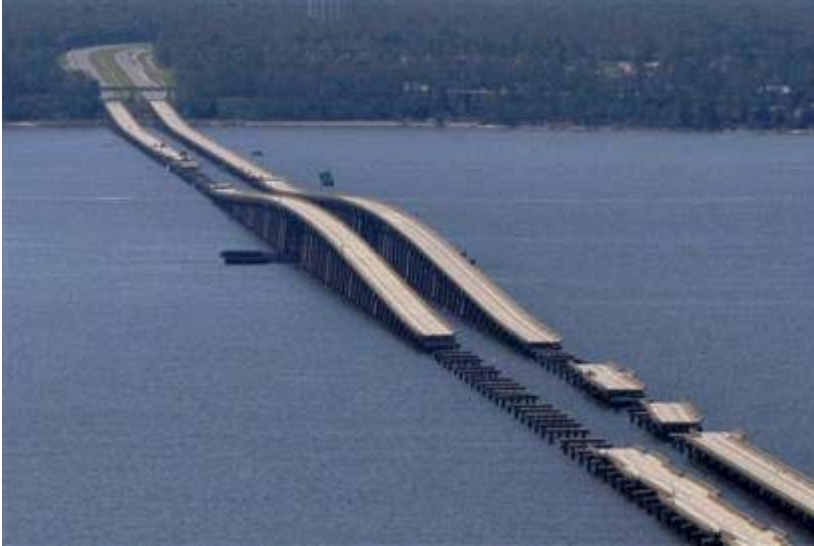
The Interstate 10 bridge that spans Pensacola Bay, is seen with sections washed away in the aftermath of Hurricane Ivan, Friday, Sept 17, 2004, near Milton, Fla
